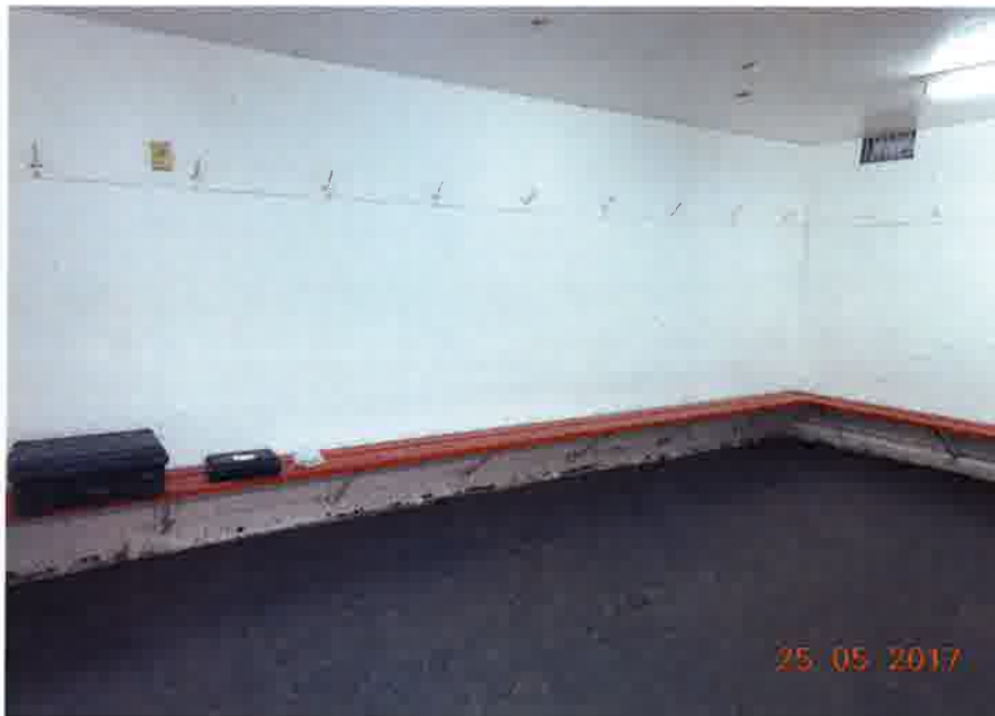
Photo 4 - Additional view of Dressing Room #4 where mold growth was observed.
