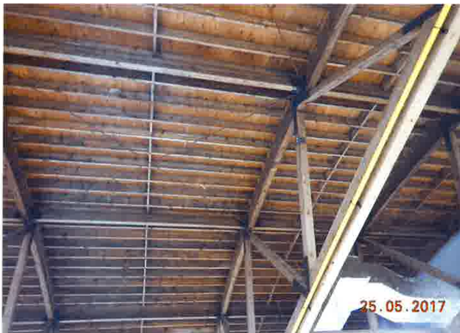
Photo 2 - Wood trusses within main arena area, where evidence of water damage and mold growth was observed.
