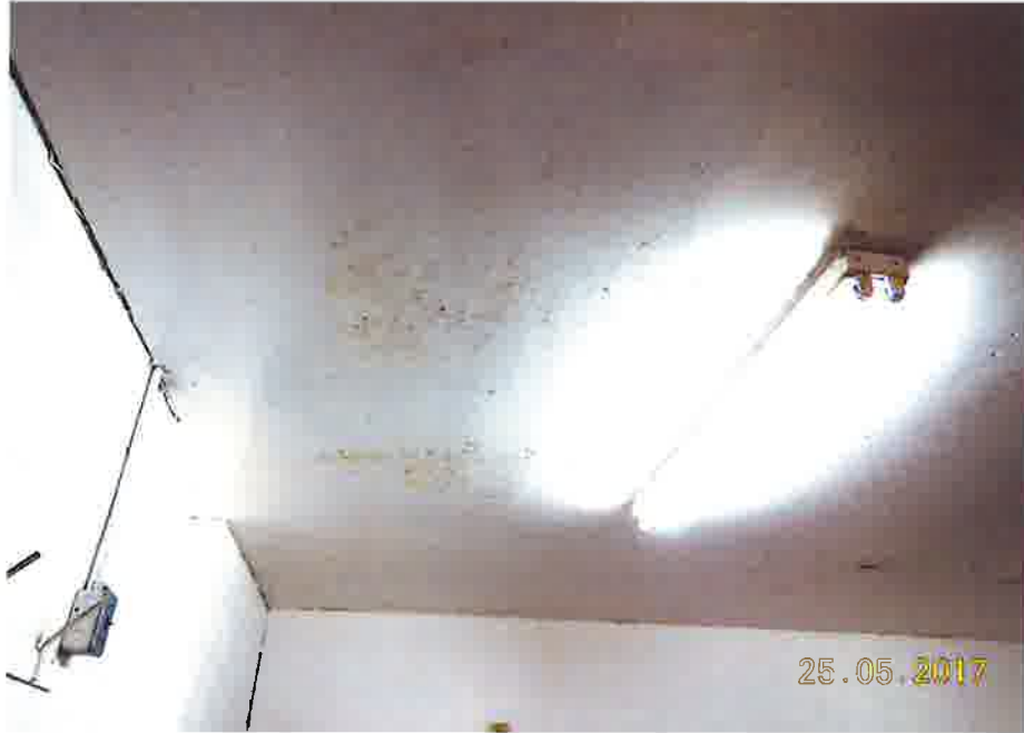
Photo 3 - Mold growth observed on ceiling of Dressing Room # 4.
