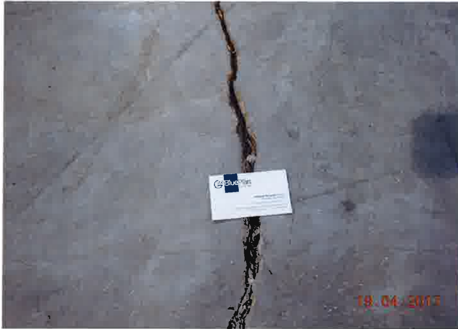
Photo 11: View of wide crack in floor slab.
