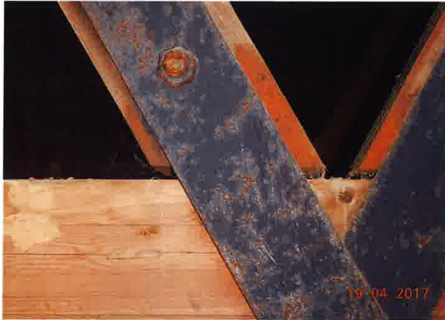
Photo 13: View of gap between webs and bottom chord of trusses.
