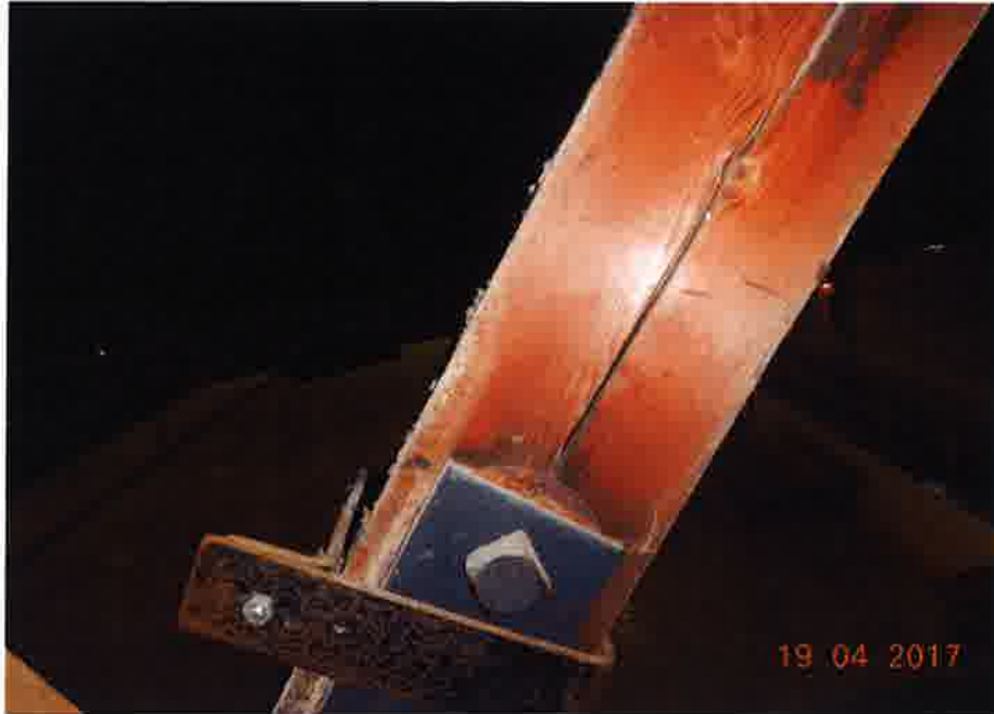
Photo 9: View of typical split in truss web member.
