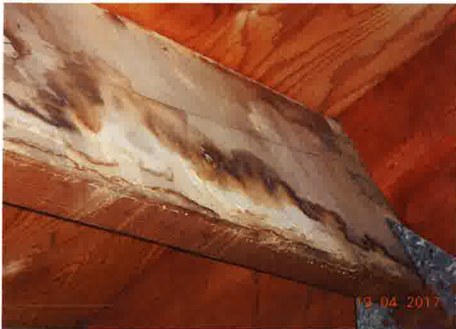
Photo 16: View of typical moisture damage and mold on roof purlins.
