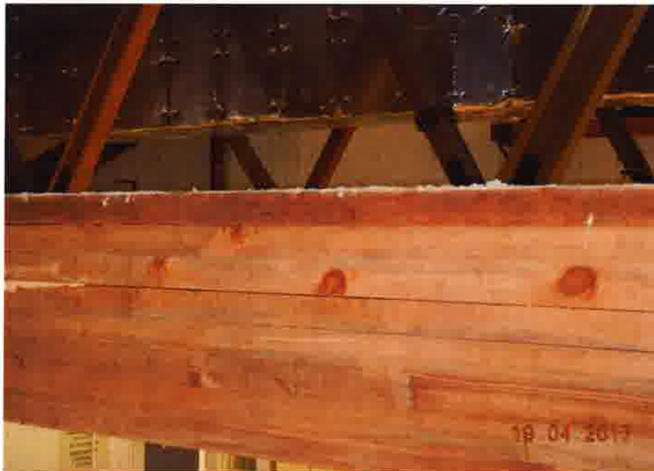
Photo 10: View of delaminating of bottom chord.
