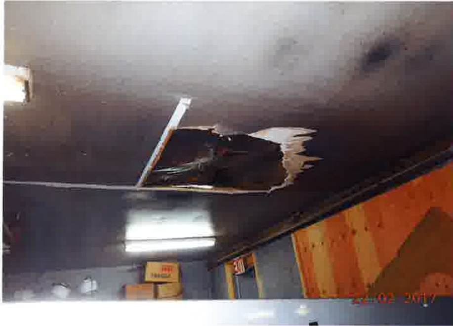
Photo 5: View of moisture and mold located in Zamboni room ceiling.
