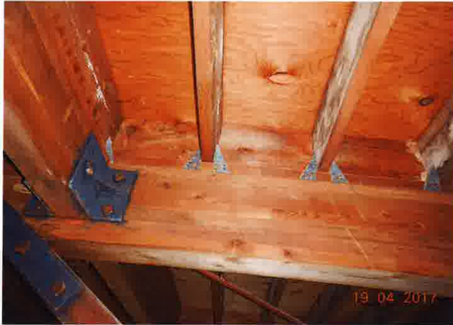
Photo 15: View of typical mold on purlins.
