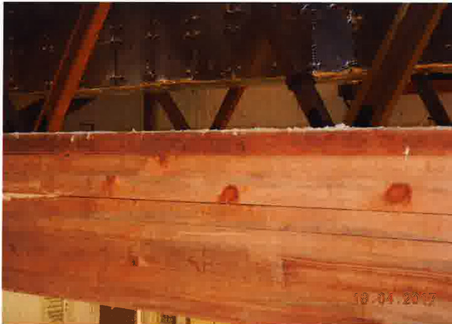
Photo 12: View of delaminating of bottom chord.
