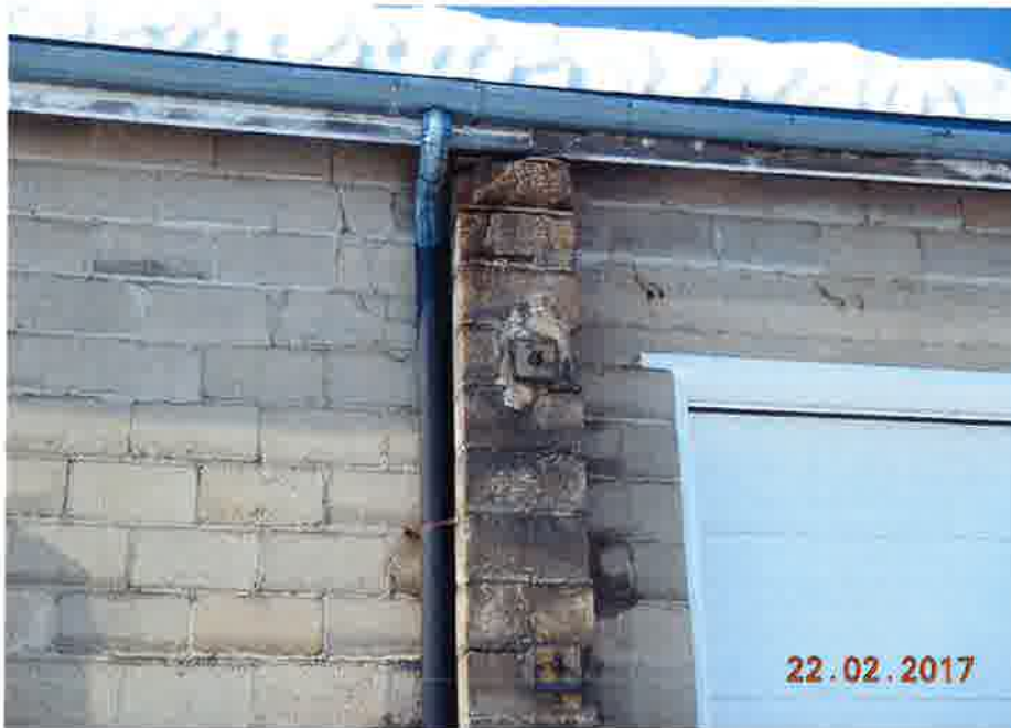
Photo 6: View of typical pilaster deterioration.
