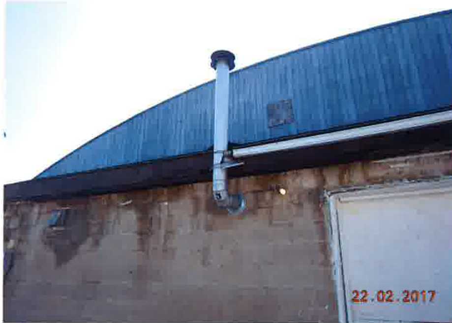
Photo 7: View of missing eavestrough and rotting fascia board.
