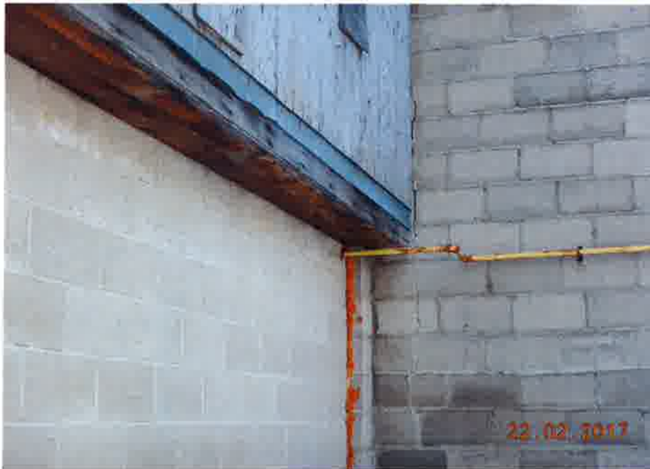
Photo 8: View of rotting soffit located outside the Zamboni room.
