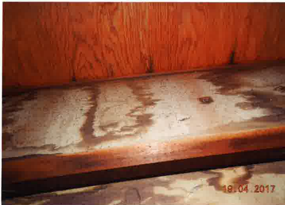
Photo 14: View of typical moisture damage on roof purlins.
